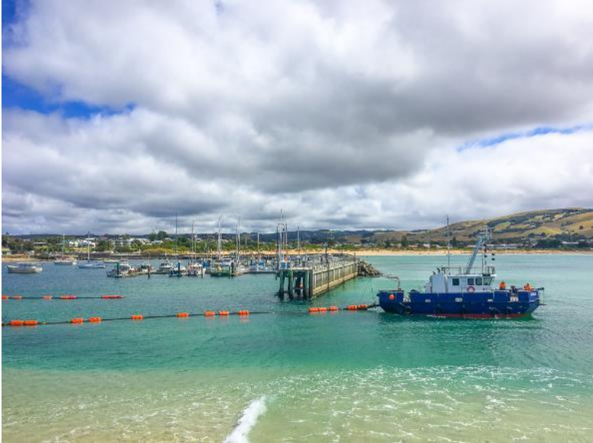
The dredge at work at the entrance of Apollo Bay. Days of work to re-open the harbour!
